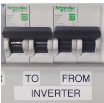
*To Inverter Breaker
