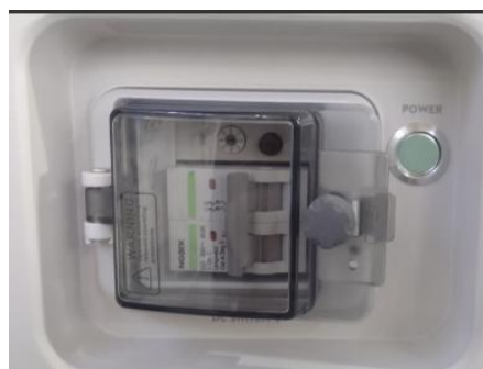
*Battery supply breaker
